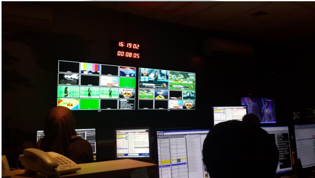
Gambar 3.6 Control Room Kompas Sport
