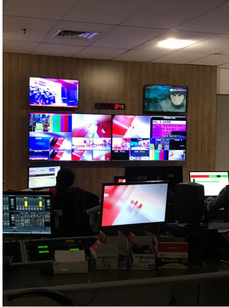
Gambar 3.14 Control Room MNC News
