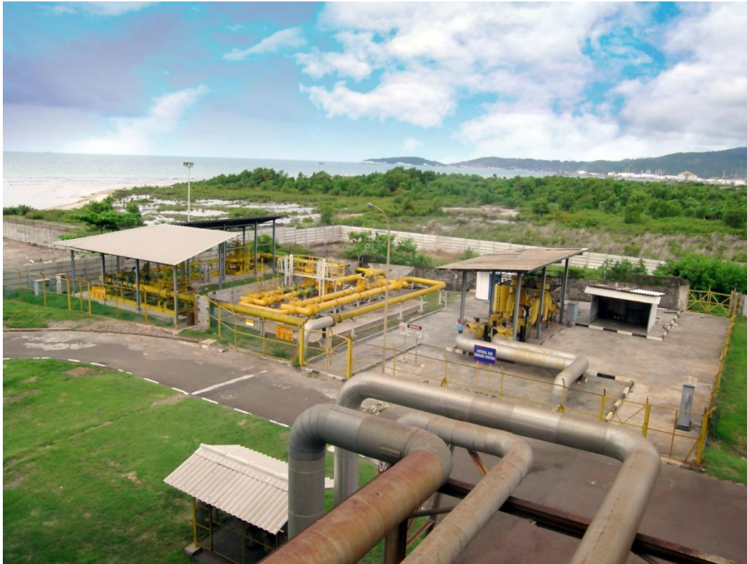
Gambar 2.9 Pipa Gas PT KDL
