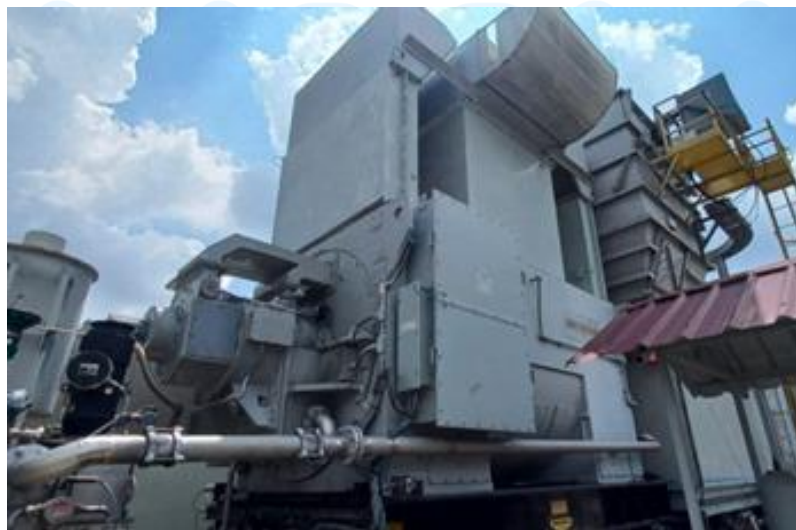
Figure 1. 1 Overhaul Generator 30 MVA, 11.5 kV
