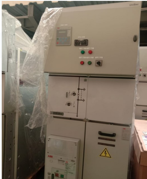
Gambar 2.2 Medium Voltage Cubicle (Panel)
