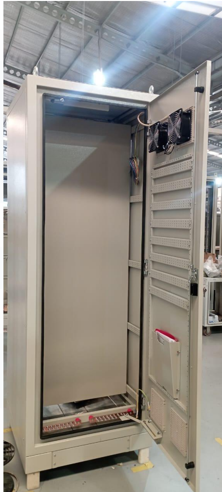
Gambar 3.12 RTU System Cabinet (Rear)
