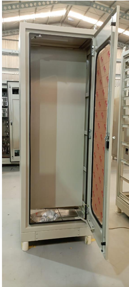
Gambar 3.13 RTU System Cabinet (Front)
